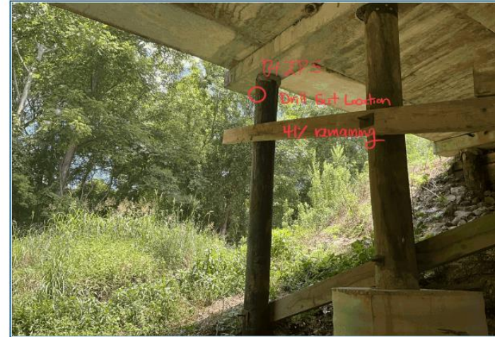
Photo 28 (7/15/2026 8:31:12PM): BT2P5 Critical Finding pile.
