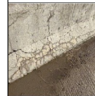
Rating 1 Delamination West End
