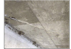
Deck Underside Diagonal Cracking with Efflorescence
