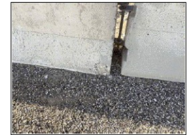
Rating 2 Spall West End
