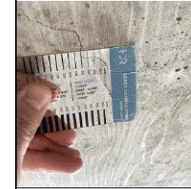
Roadside Longitudinal Cracking 0.013 IN
