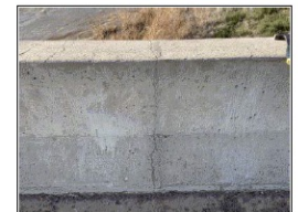
Concrete Railing Vertical Cracking
